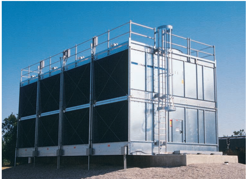
Four-cell NC Class cooling tower serving a municipal power plant.
