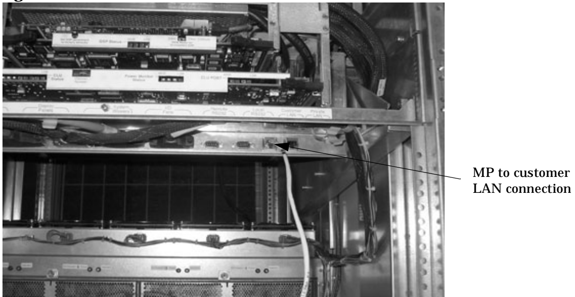
Figure 3-38 MP LAN Connection Location
